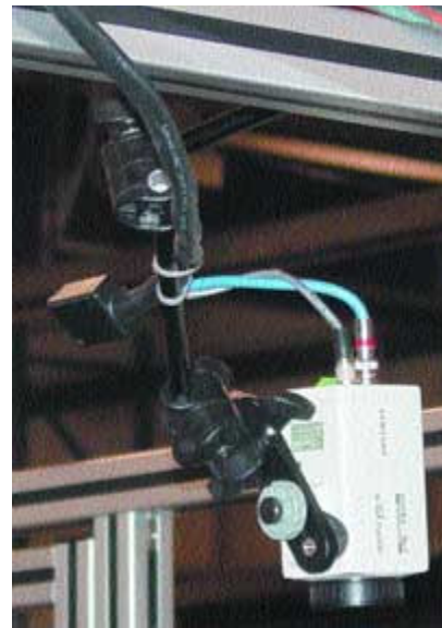
Camera is aimed at a potential problem location. System replays archived video in a choice of four different speeds.
